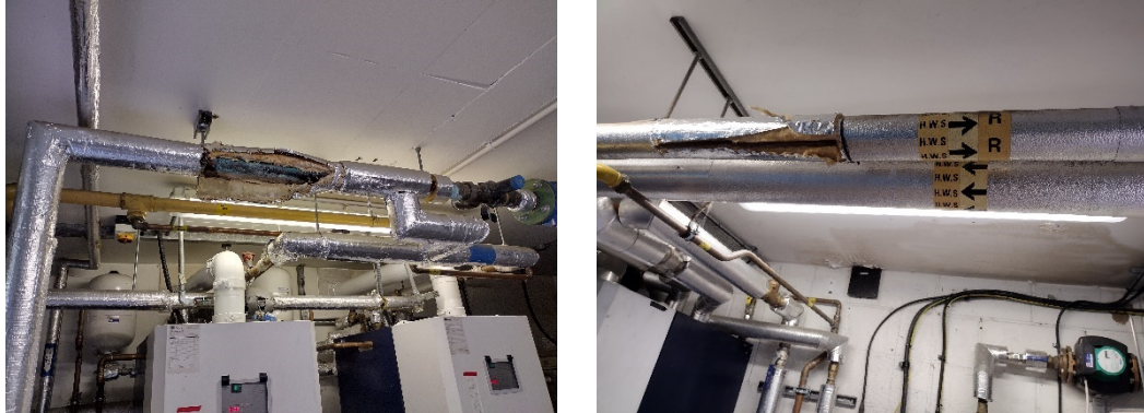
Figure 13: Examples of heating pipes insulation in Beaumont Court and Stocks Court
